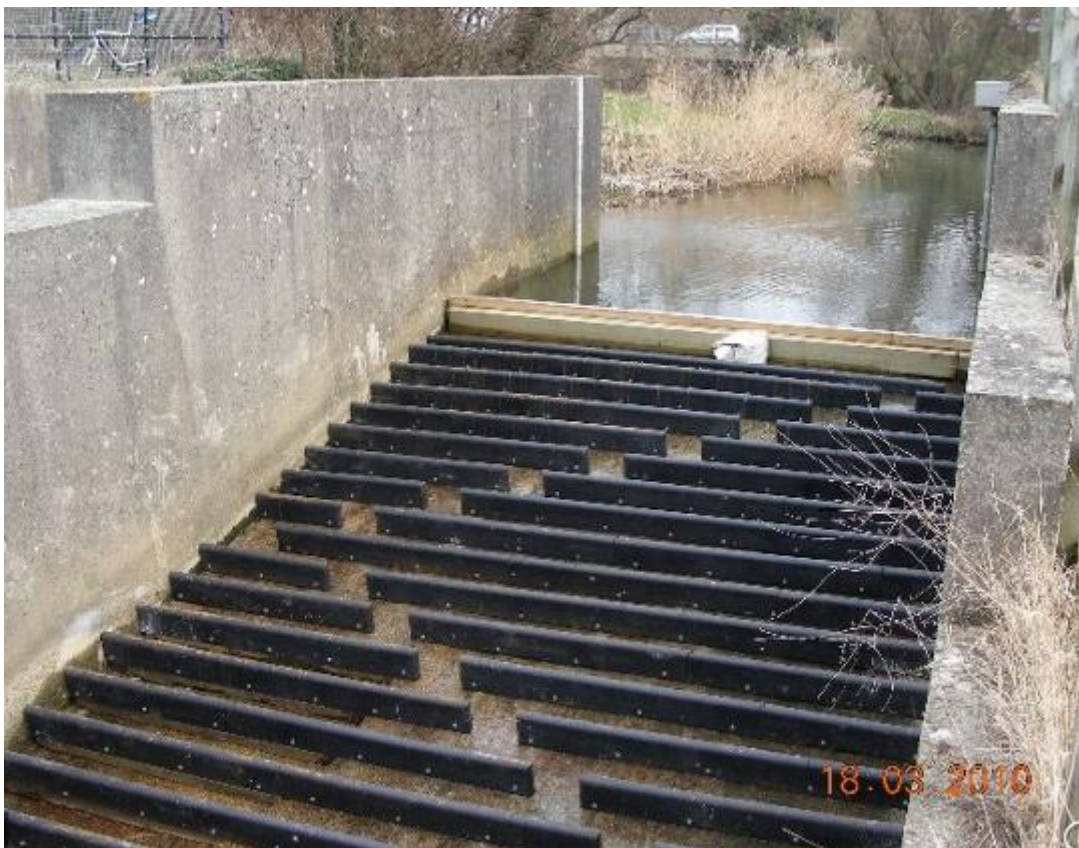
Photo 4. Plastic baffle pass installed on an EA owned crump weir.
