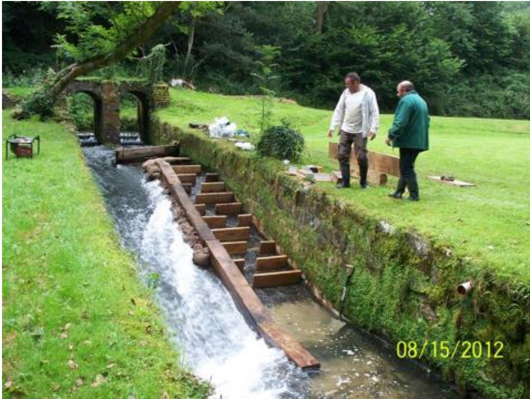
Photo 3. Low cost baffle system constructed in oak on the Costers Brook in West Sussex.
