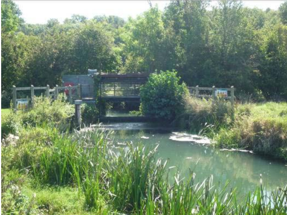
Large EA owned structure. The exact purpose and requirements for this structure should be explored as it severely restricts habitat recovery and fragments fish populations
