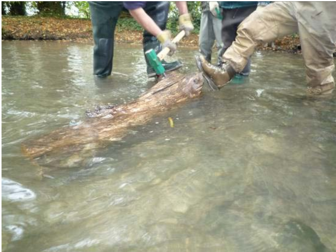
A piece of LWD being secured to the river bed with steel re-enforcing bar. The deflector is configured to encourage bed scour to free up loose gravel for spawning
