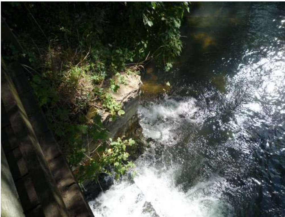
Rag Mill Weir with the breach in the wing wall evident. Lowering the impoundment will take pressure off the leak and improve habitat.
