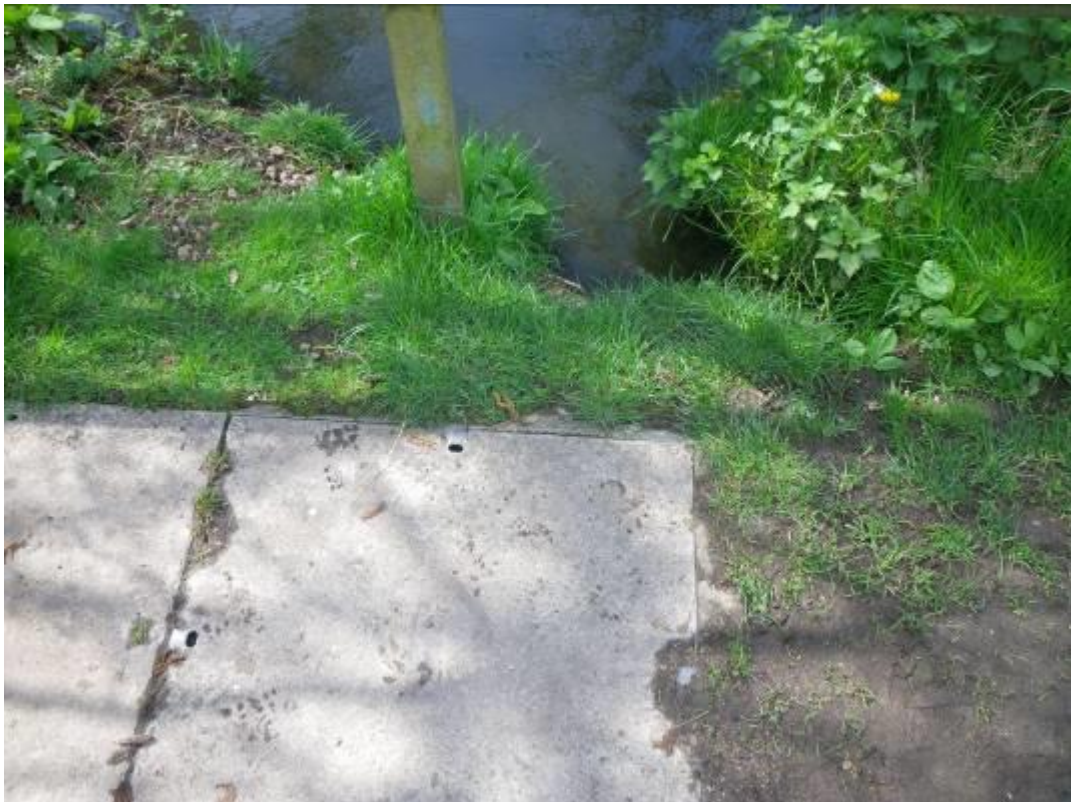
Photo 8. Manhole cover on the canal tow path above a hydraulic connection between the canal and river. The impounding structure in the river may be linked with water supply to the canal, or this may simply be a drain for excess water in the canal pound.
