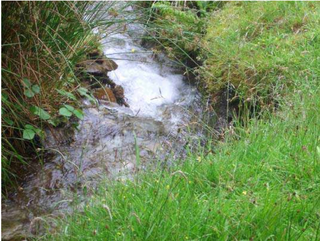
A typical little plunge pool. Note the eroded geotextile on the RH bank.
