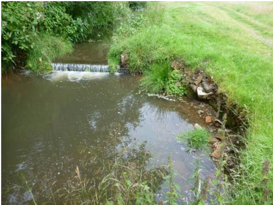
Photo 2 Bank erosion and channel widening caused by flow patterns generated by the weir in high flow events.
