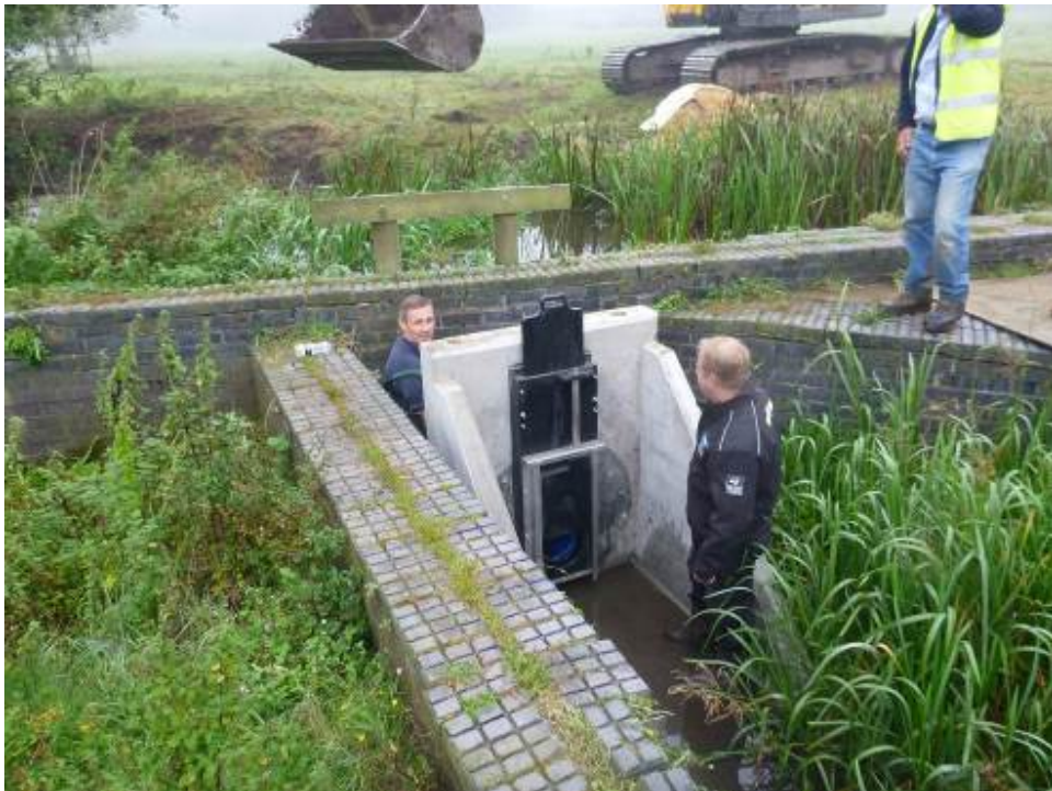
Photo 13 Installing a pre-fabricated penstock sluice at a lake inlet from the River Glaven, Norfolk.
