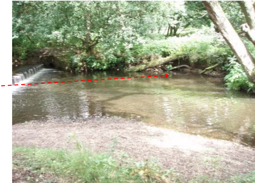
Photo 2 High flows are directed against the eroding bank by the pipe weir
