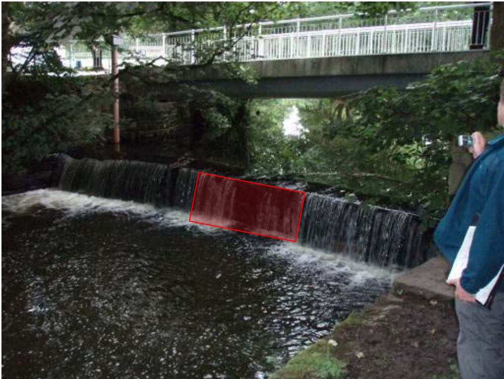
Photo 5 The large weir near the cricket pitch. The simplest solution to improve fish passage and upstream river habitat would be to remove a central section (as indicated). Entire removal of the weir should be considered as well.
