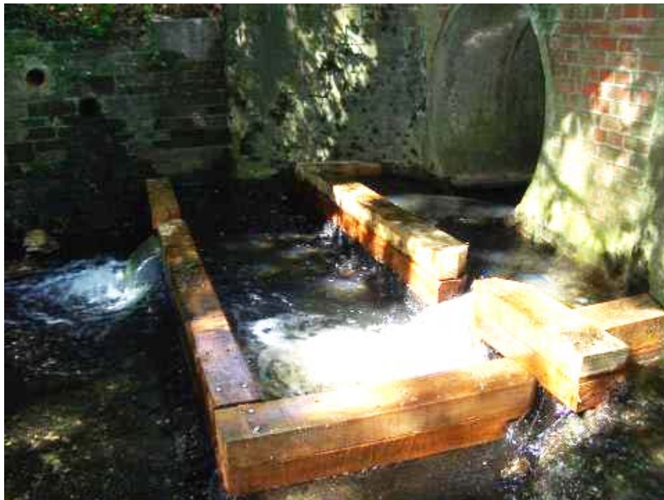
Photo 7 Timber baulks with notches used to create an easement at a barrier to fish migration (Sussex Ouse).
