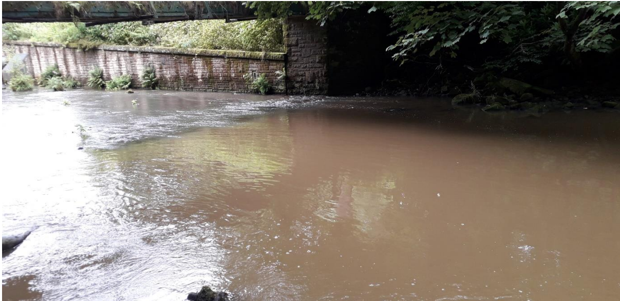
Figure 19: Sediment photographed below Jumbles Reservoir dam wall.
