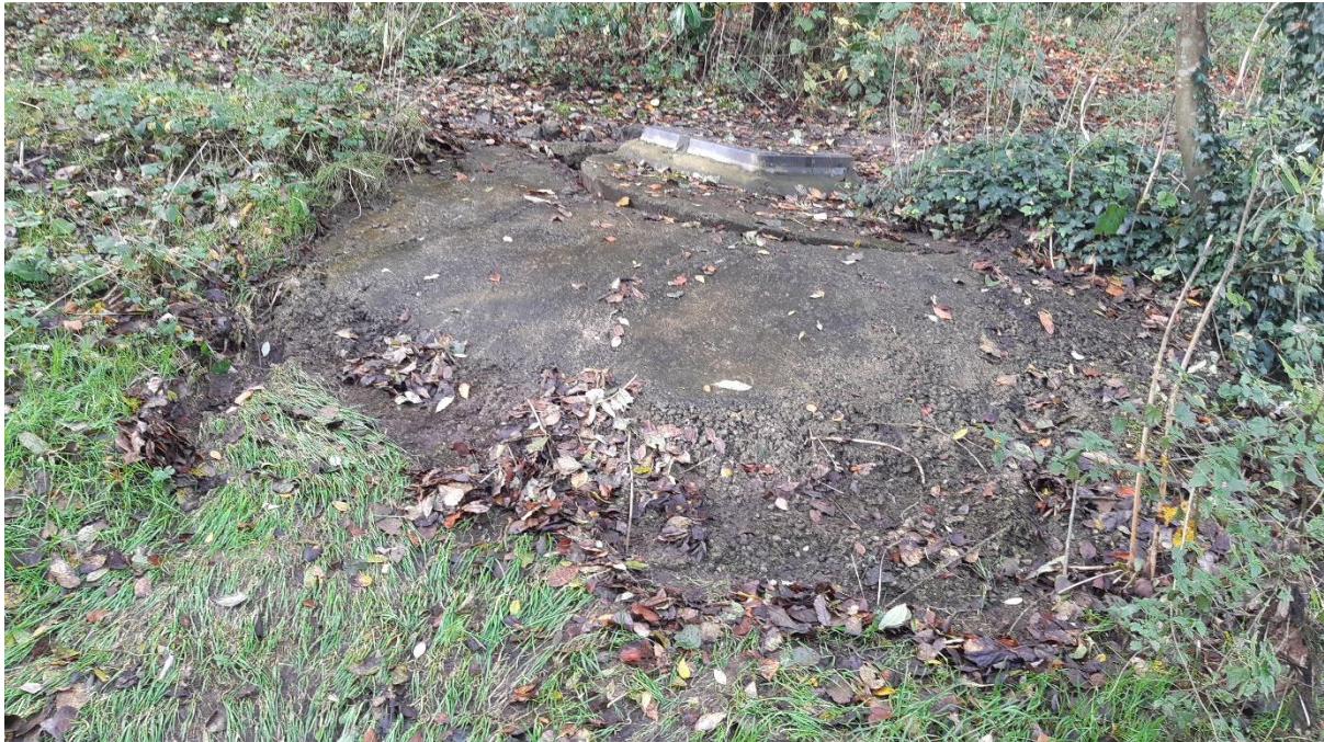
Figure 11: Raised drain cover with apparent split in the concrete casing. Note flattened grass below the concrete mound indicating a recent overflow into the river (which is just outside the frame, below the lower edge of the picture).
