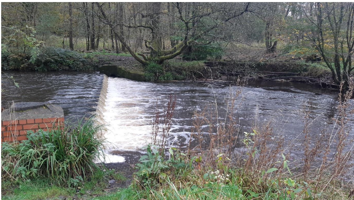
Figure 15: This weir apparently exists to stabilise and protect the services pipe which crosses the river at this point.
