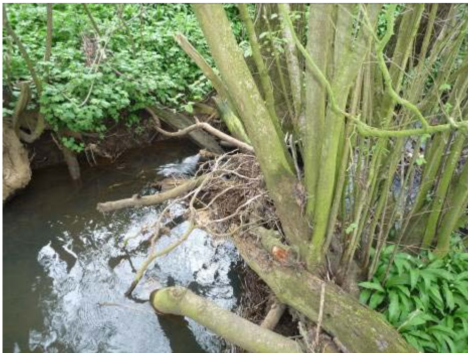
Small debris dam on the adjoining tributary. This dam presents no difficulty for migrating trout
