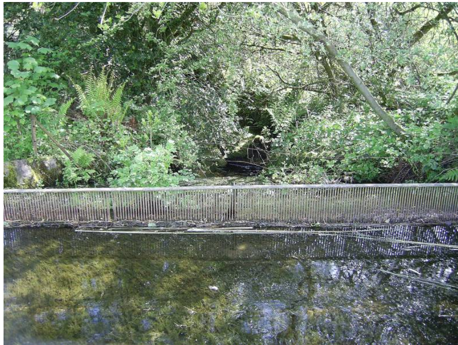
Figure 3: Corroded fish screen
