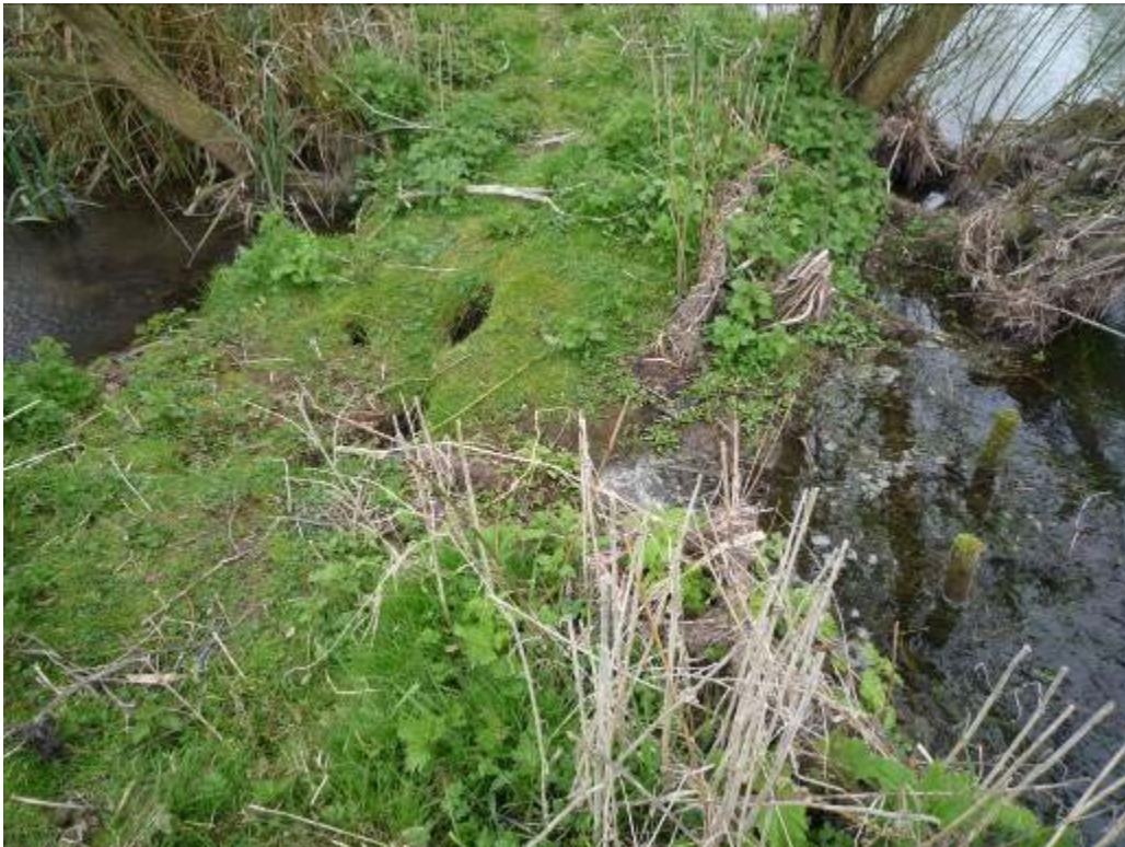
Main river bank a few meters upstream from the carrier take-off point. Hugely vulnerable to a major breach.
