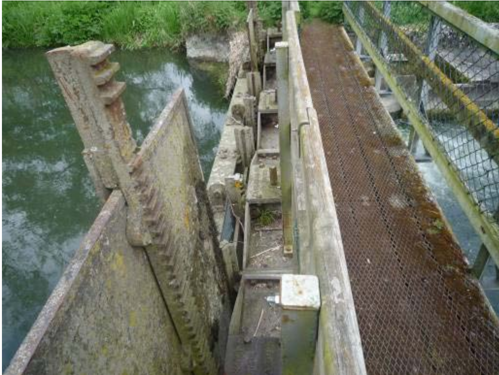
Two Hatches at Gunville closed presumably to maintain upstream water levels
