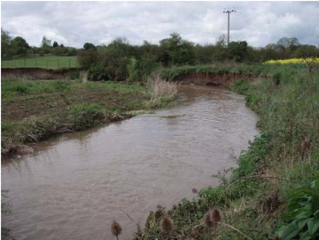
Photo 6 Downstream limit of Site 1. The eroding bank could be protected here, maybe by reveting the toe of the bank with willow logs or brushwood, but changing the land use on the right bank to woodland to increase bank resilience would be required for a longer term solution.
