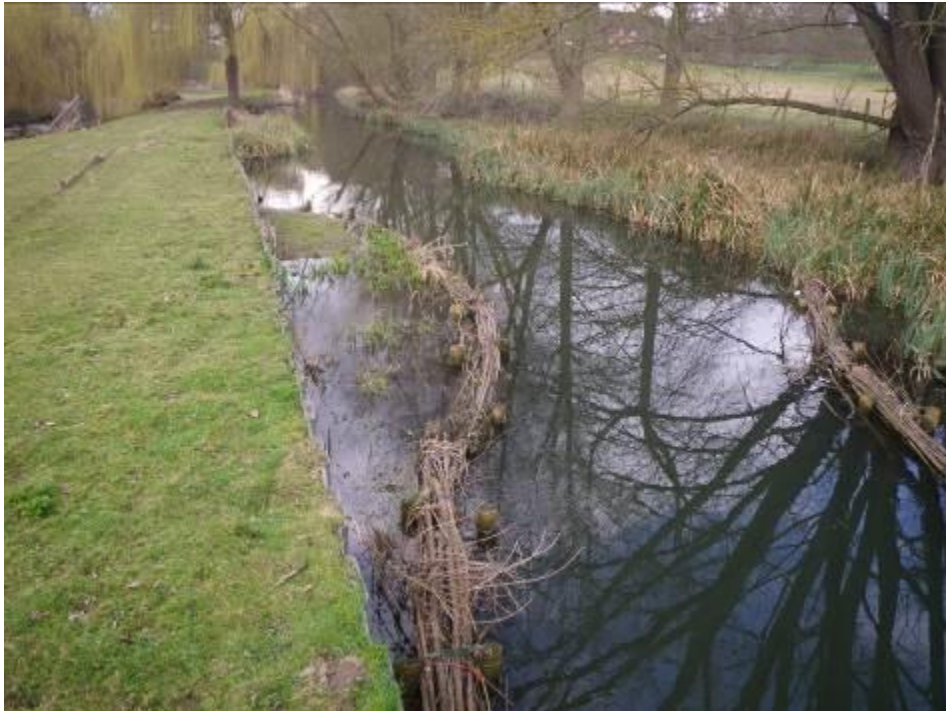
Photo 4. Mill leat. Some excellent attempts have been made to add some sinuosity to the Mill leat channel; however, the revetments require more brushwood, or gravel backfill with planting and possibly tree work to let in more light and maximize marginal emergent plant growth potential.
