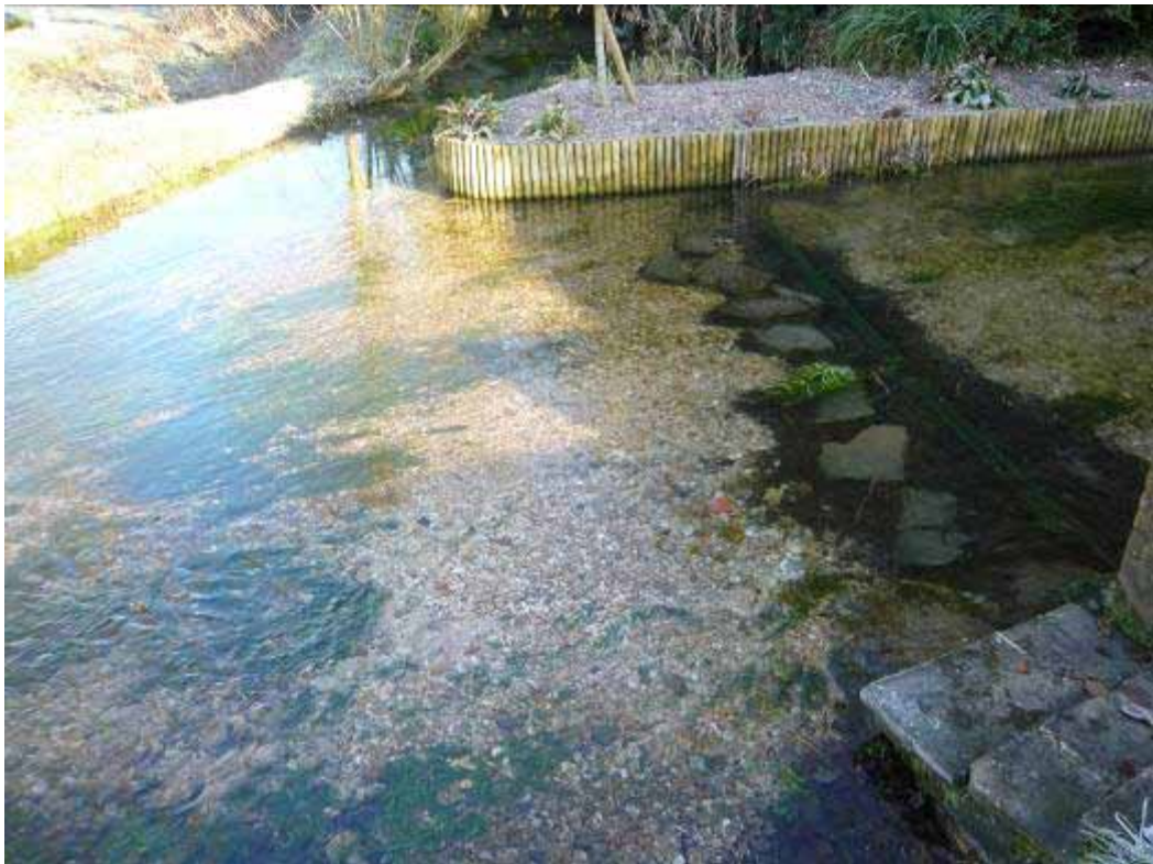
Remains of an old stone weir now flattened. Note the hard revetment on both banks
