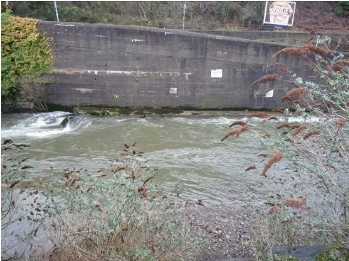
The Afan just above Port Talbot where the channel is reveted with steep sided brick and concrete walls.
