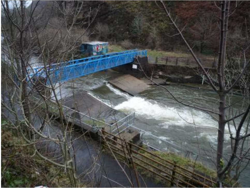
A crump-style flow-gauging weir. Is this an issue for sea trout migration during a low flow summer?
