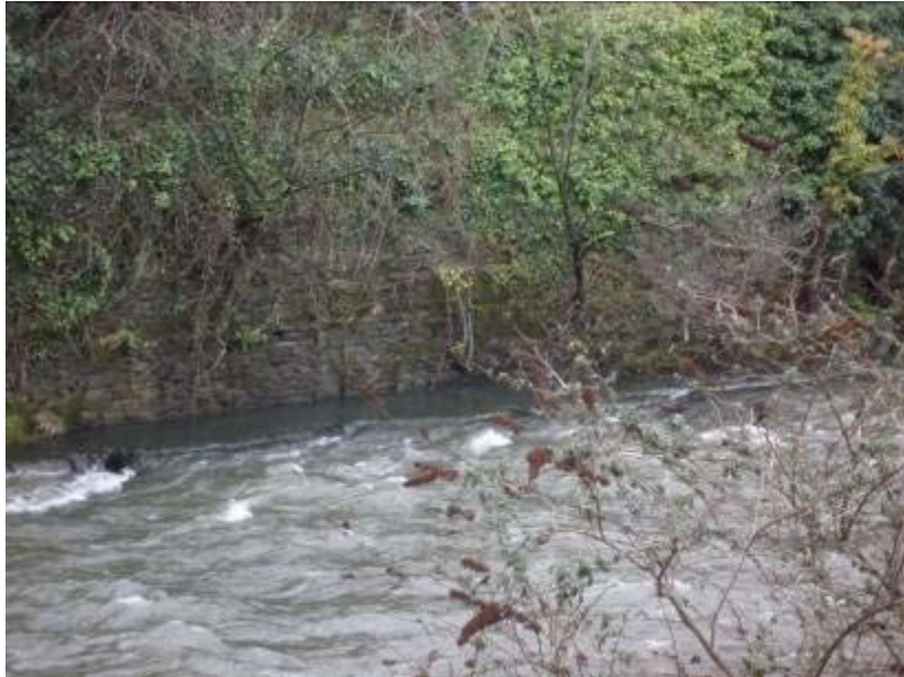
Exposed major sewer pipe running within the river channel
