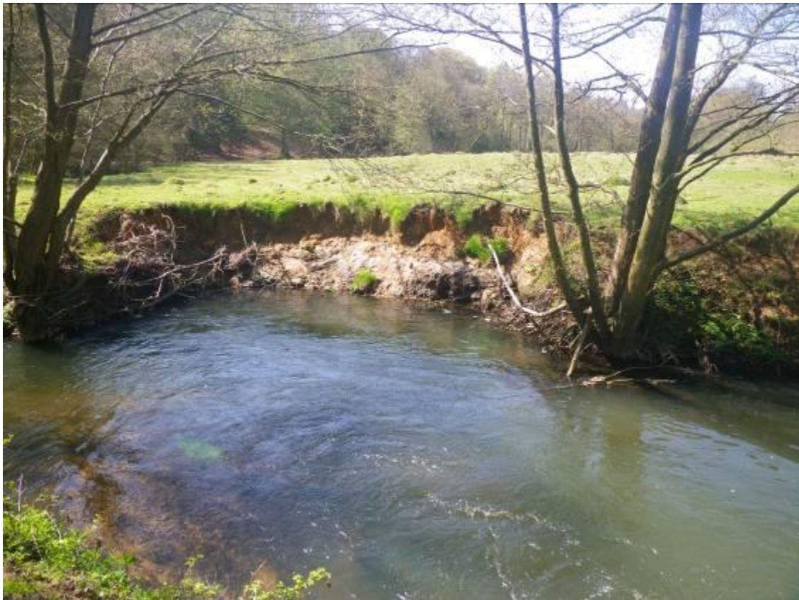
Photo 5. Erosion caused by winter back eddy impacting on a heavily grazed bank
