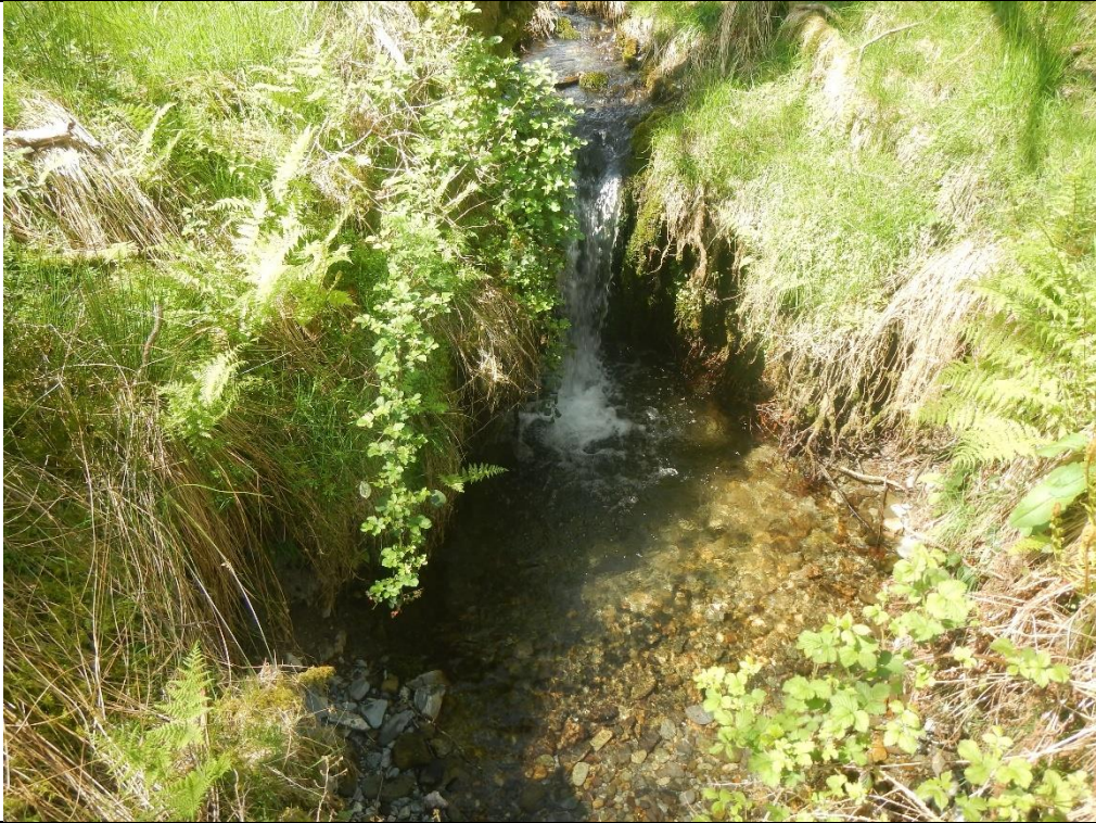
Figure 8 (56.187878, -4.440153). The head-cut nick point in the channel d/s of the culvert – created by starvation of sediment supply to the channel and, almost certainly, dredging d/s.
