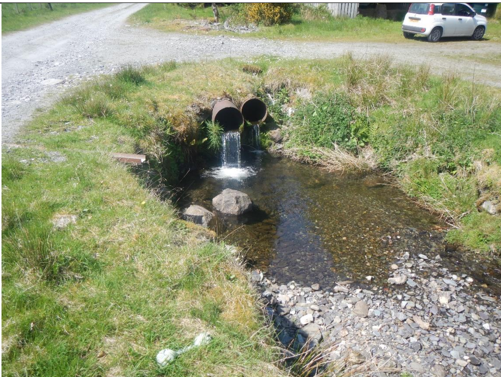
Figure 3. Perched culvert pipes created a series of major barriers for fish. The energy dissipation at the fall did facilitate some retention of the gravels that passed through, but these structures are highly detrimental and should be replaced with much larger, partially sunken structures to facilitate free passage of fish and sediment.
