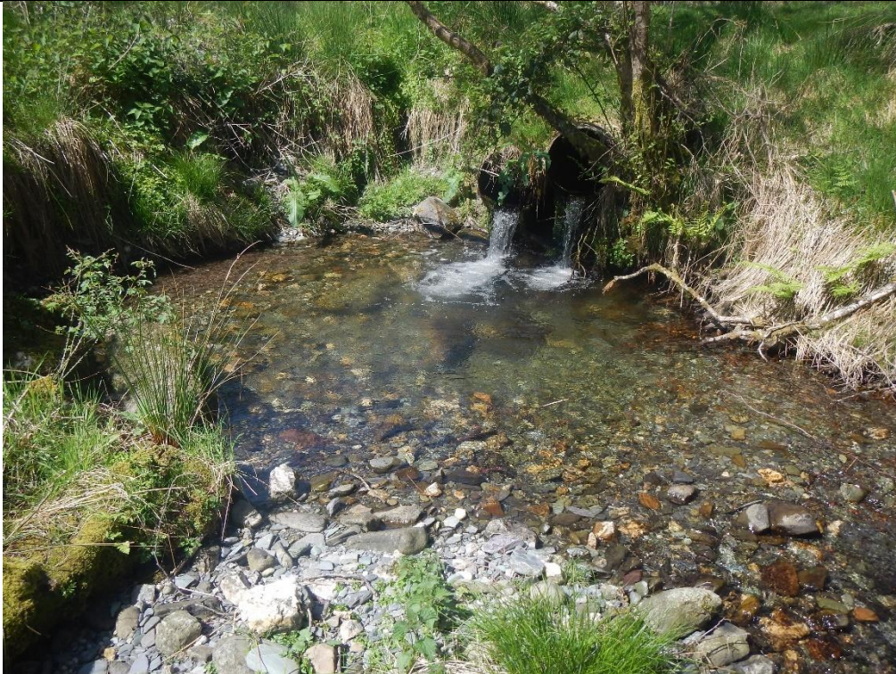
Figure 7. Perching at the d/s side of the culvert pipes.
