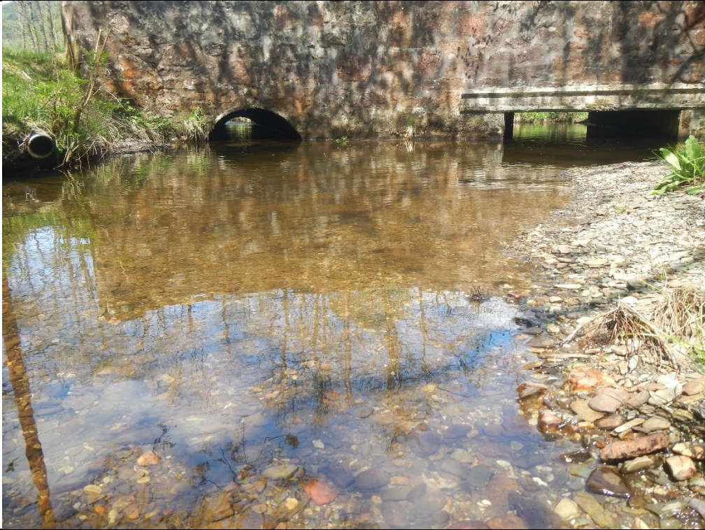
Figure 19. The somewhat undersized road culvert. This should be maintained clear to ensure free fish passage at all times – not just during spawning times.
