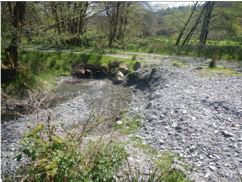
Figure 6 (56.187853, -4.44035). Another undersized and now significantly perched culvert. Note the ongoing sediment maintenance burden created by inappropriate watercourse crossings, with the entrained coarse sediment having to be regularly excavated.
