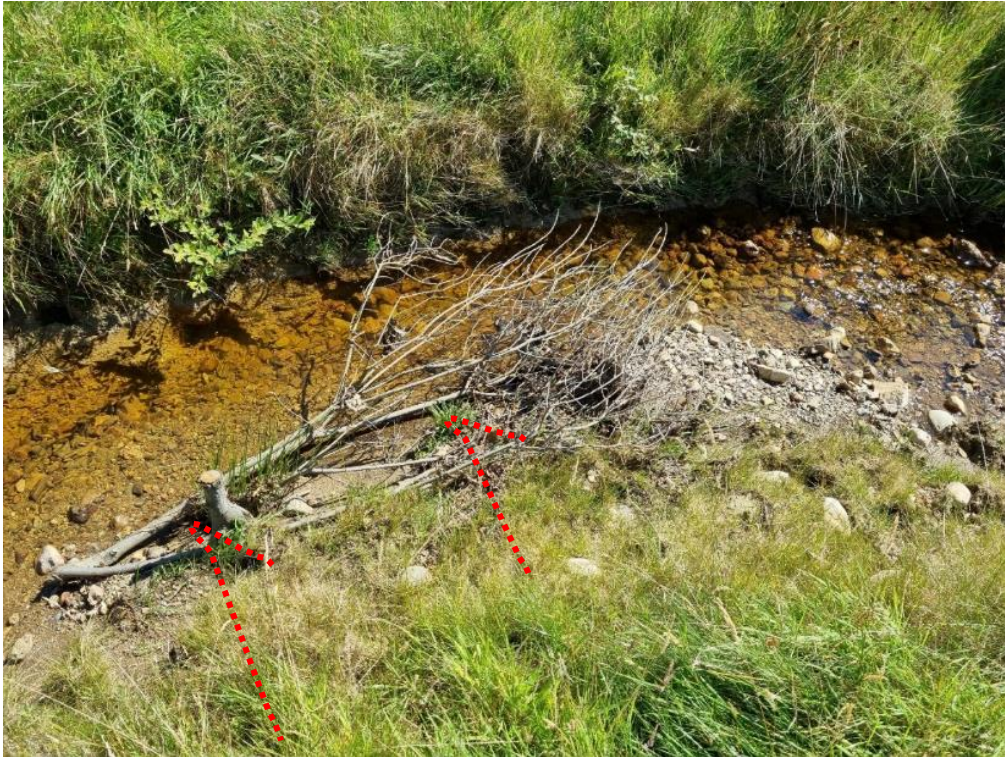
Figure 36. Willow secured with two live willow pegs (red dashed lines), created from forked branches, that were driven into the bed on a slight upstream angle. Although slightly obscured in the picture, the pegs were driven into clefts of the right side branch (and its side branches).
