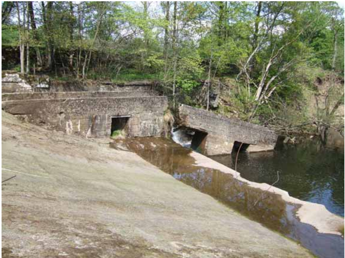
The weir is in poor repair with reinforced concrete starting to erode away, and steel reinforcement exposed.
