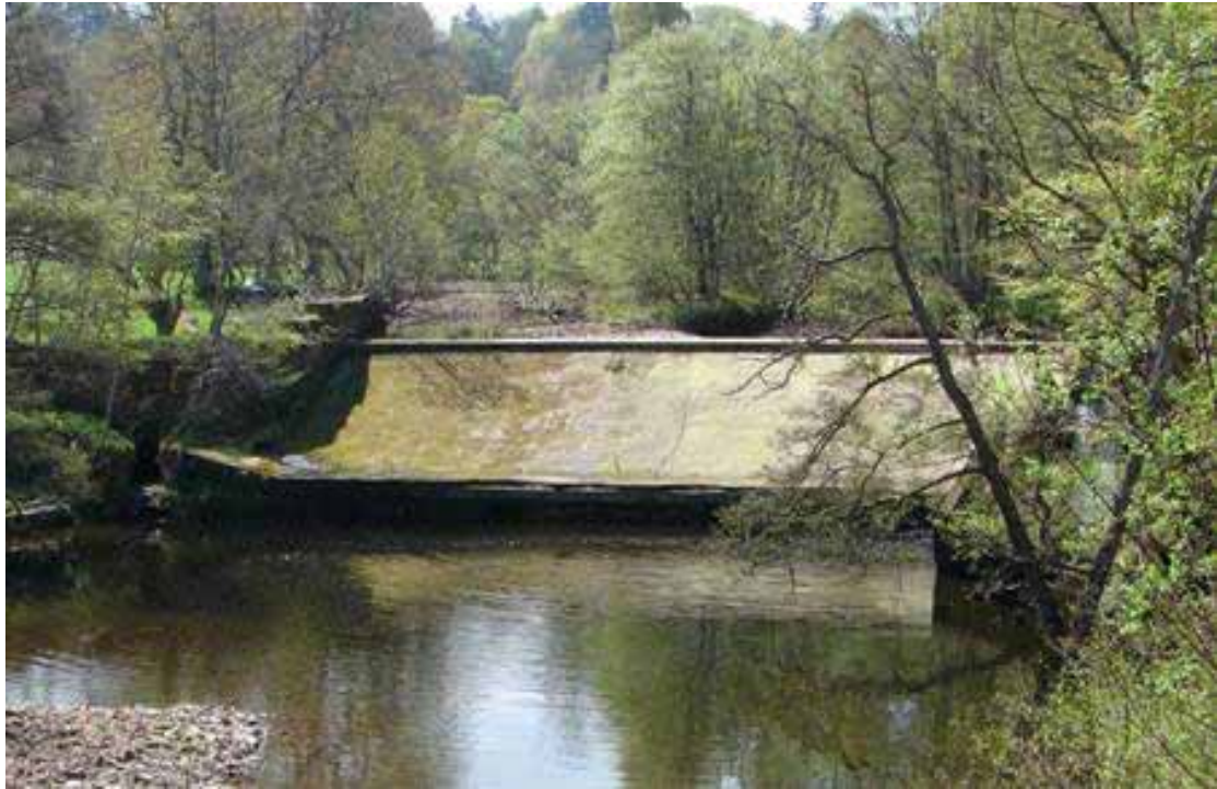
The second weir no longer serves any purpose and does not appear to incorporate an historic fish pass.
