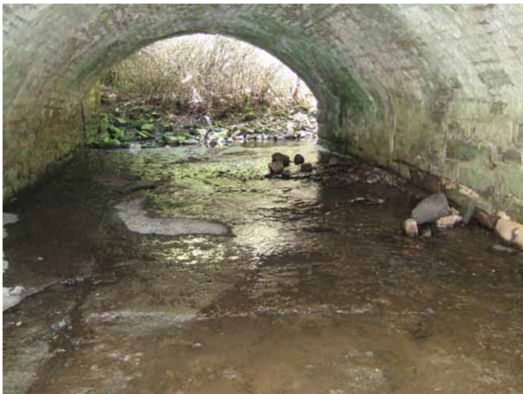
A long concrete culvert can restrict access for fish but may be easily rectified by concentrating the flow.
