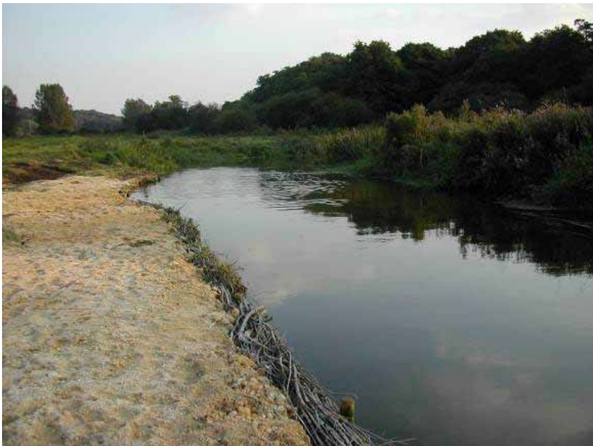
Installation of new bank using faggots and chalk backfill on the River Wensum, Norfolk
