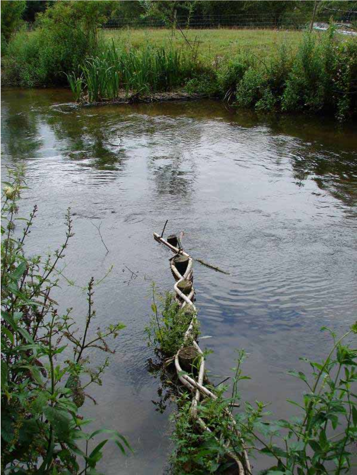
Introduction of single u/s 'natural' deflectors (single, near bank and triangular' far bank) on the Wylde in Wiltshire formed a chicanes, sending flow from one bank to another. Note set just above summer water levels.
