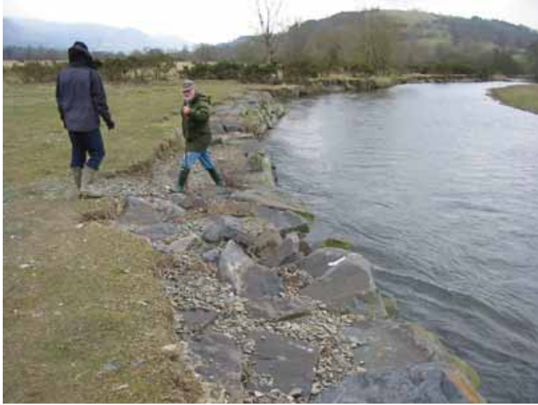
Re-instated section of stone pitching adjacent to a new gas main. The initial bank protection was eroded during a large flood event
