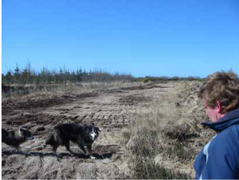
Newly excavated track with outfall from the lough to the left of the picture
