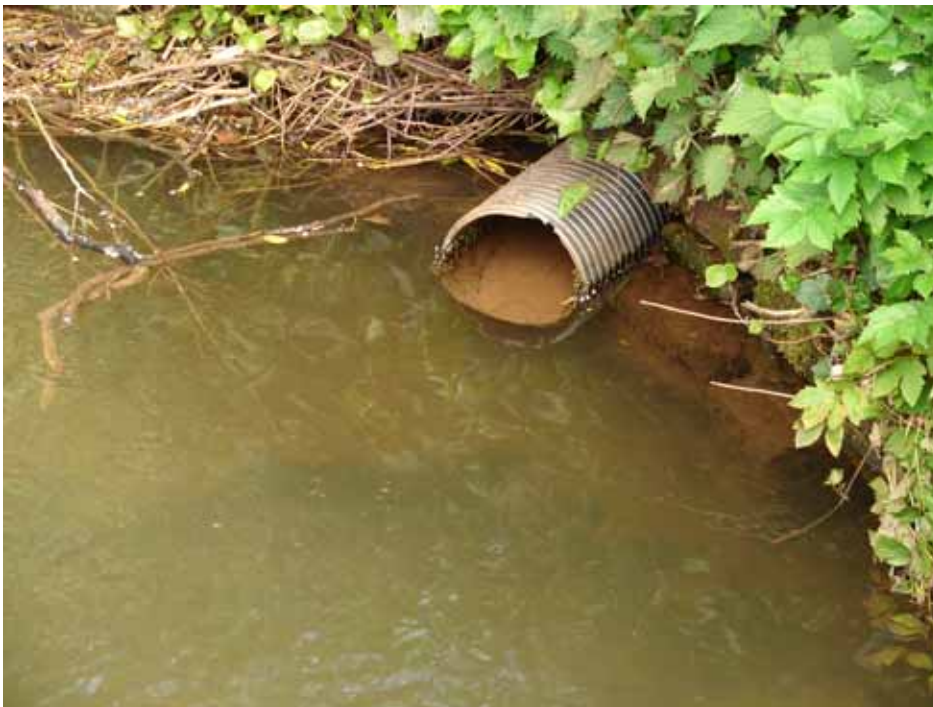
Field Drain entering brook above lake: Note silt in pipe
