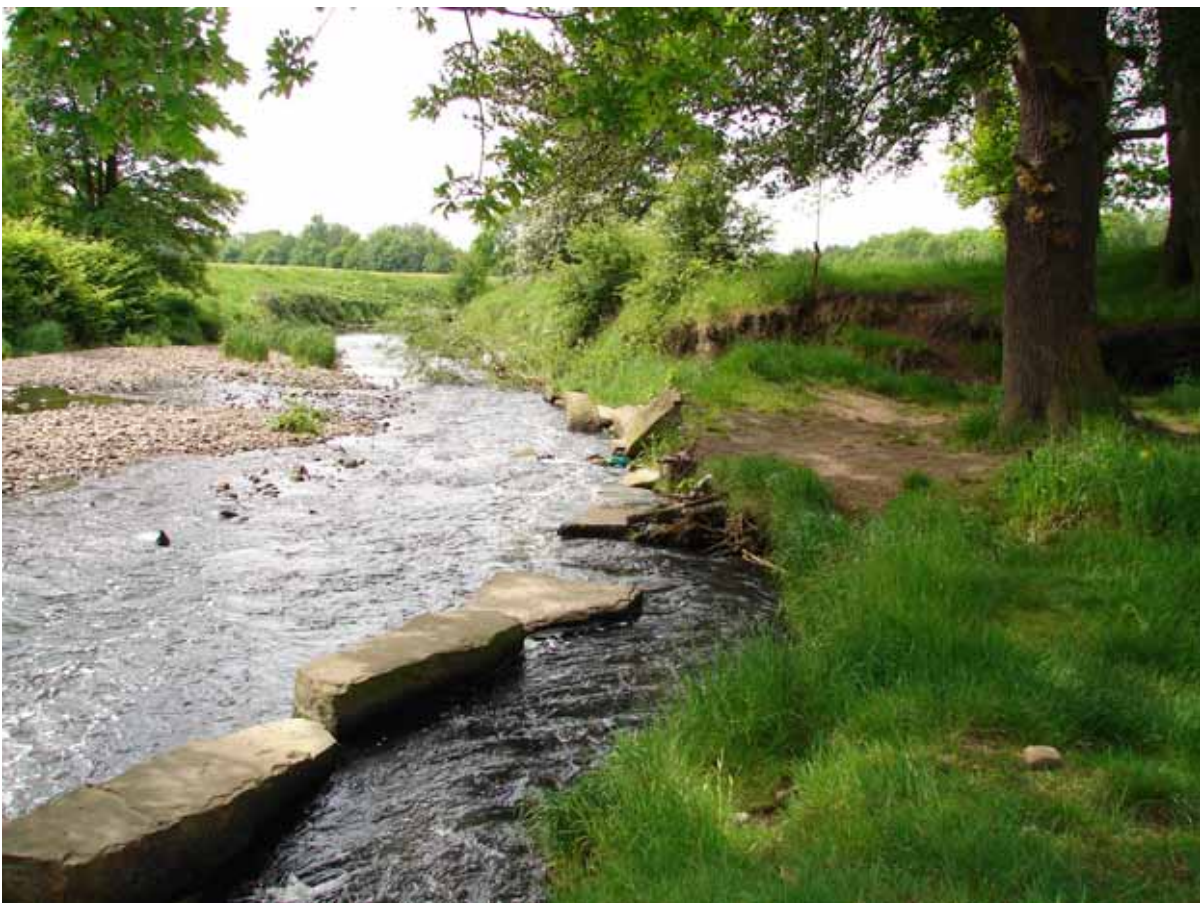
D) Failed block stone revetment, resulting erosion and major land slump.
