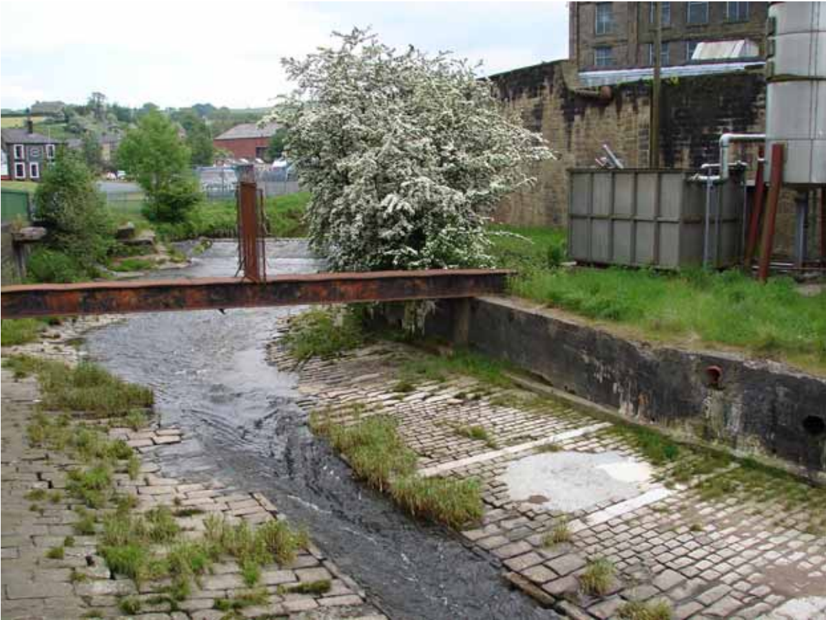
G) Relict mill structure and block stone channel upstream of Waterside Bridge.
