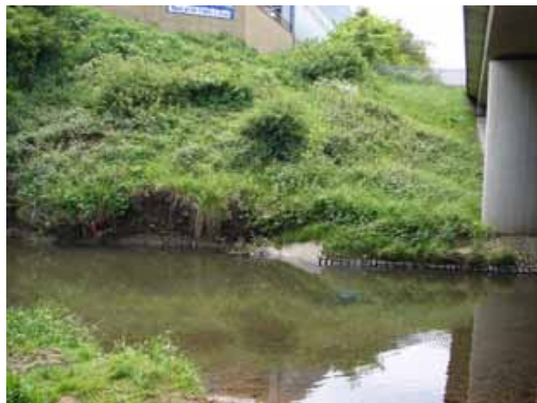
B) Erosion near M65 road bridge
