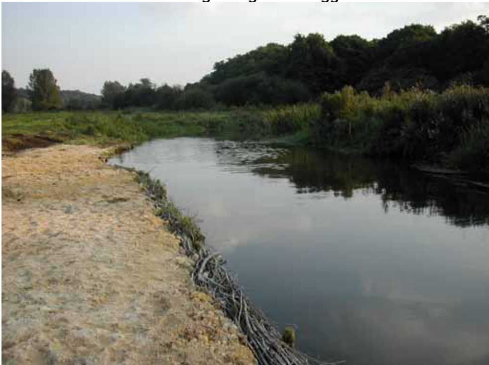
Installation of new bank using faggots and chalk backfill on the River Wensum, Norfolk (Chalk Stream)
