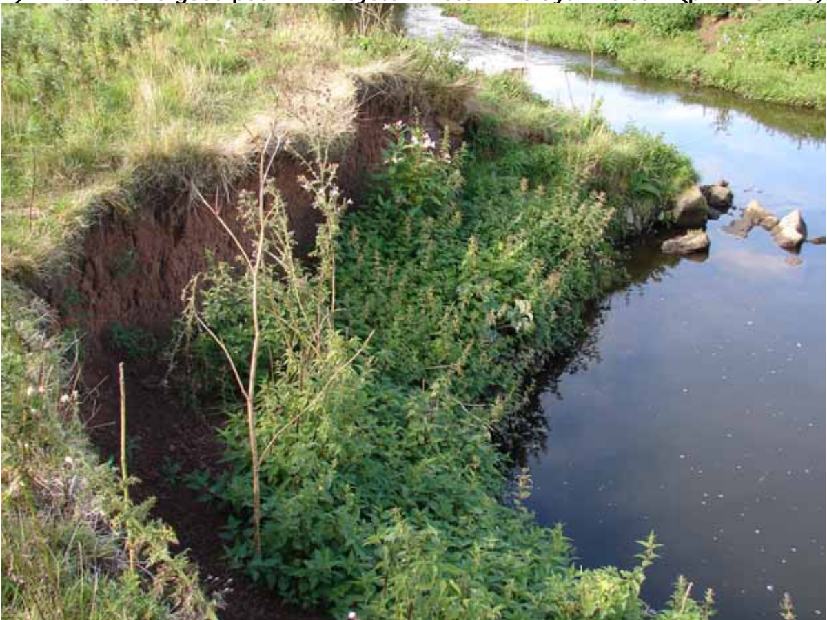
B) Major erosion on outside of bend
