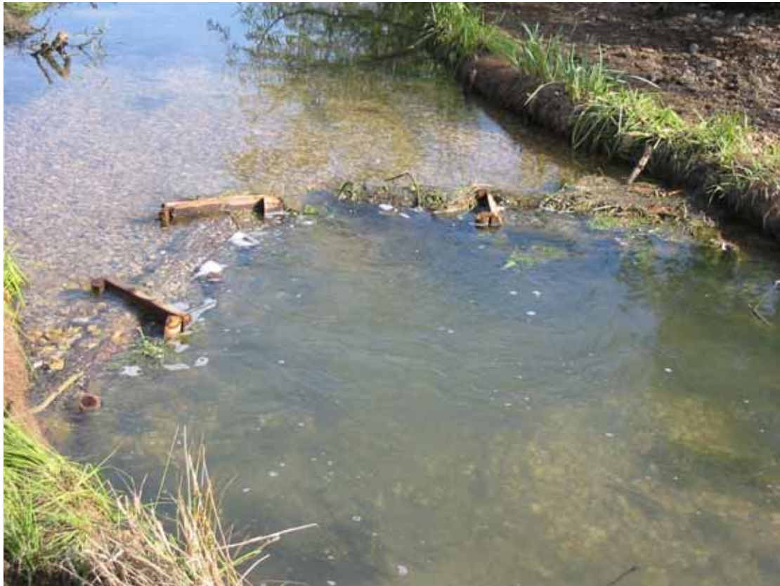
Wooden ‘v’ shaped groyne installed on gravel riffle. Note gravel backfill upstream of groyne and pool scoured downstream
