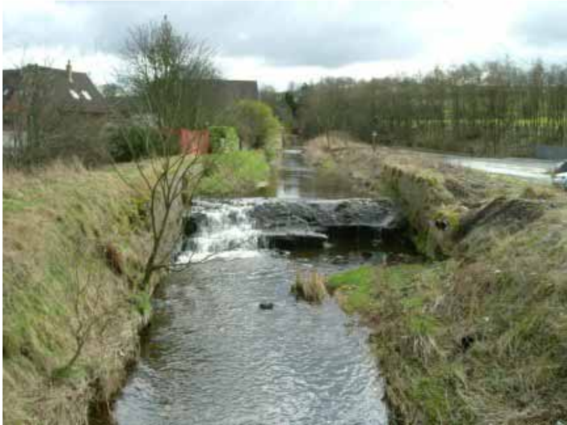
Picture 3 Redundant weir
