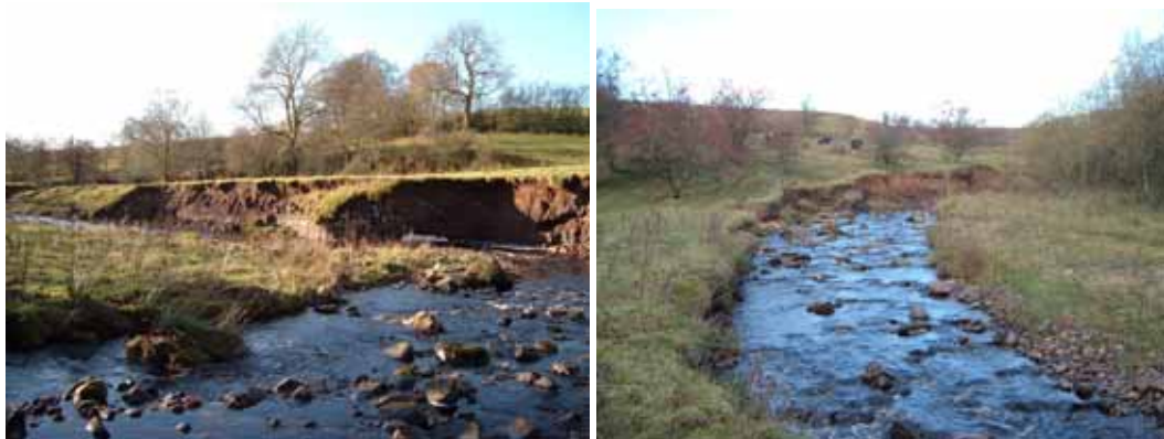
Pictures 7 & 8. The two worst areas of bank erosion, in field 13 (left) and along the lower half of field 16 (right).
