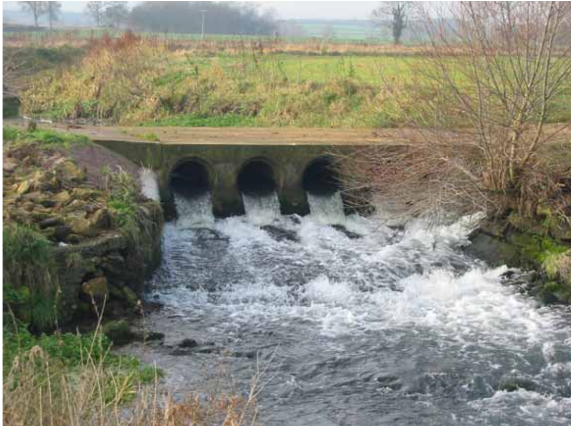
Culvert bridge showing head drop over the structure and its impassable nature
