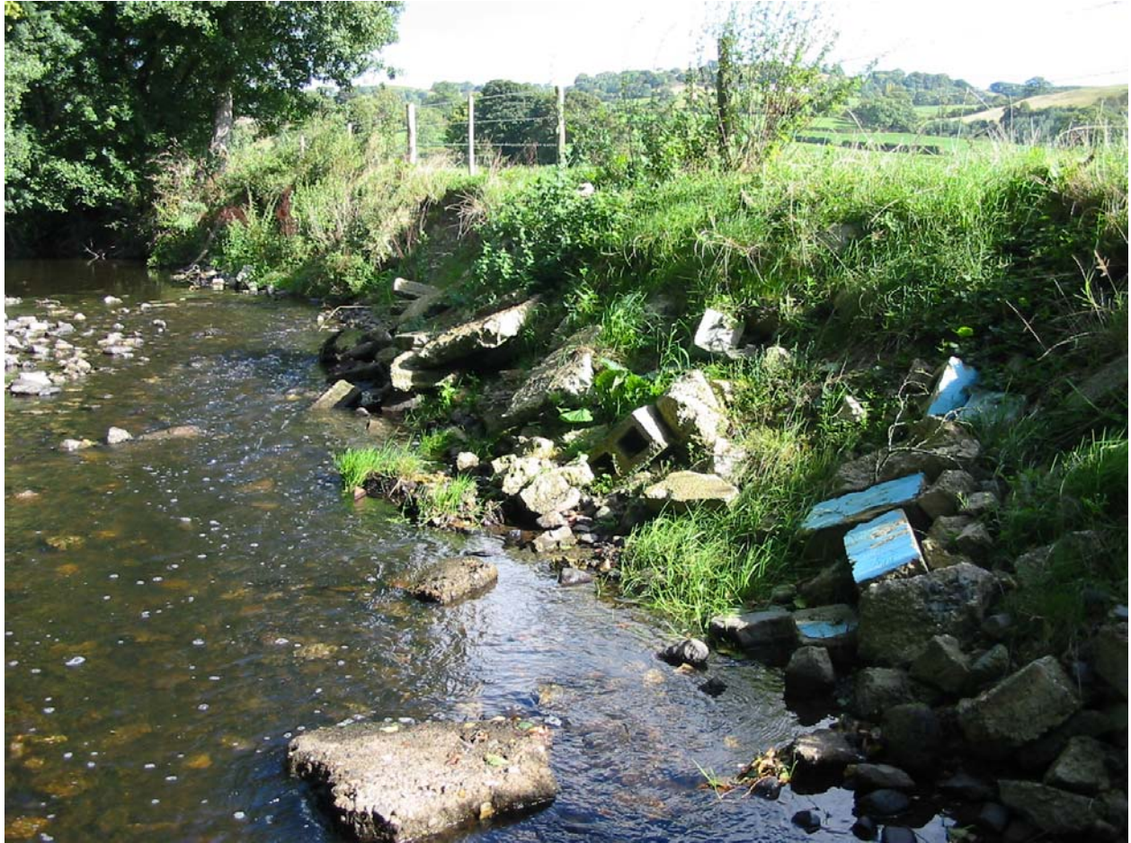
Builder's waste deposited on the LB in an attempt to stop erosion
