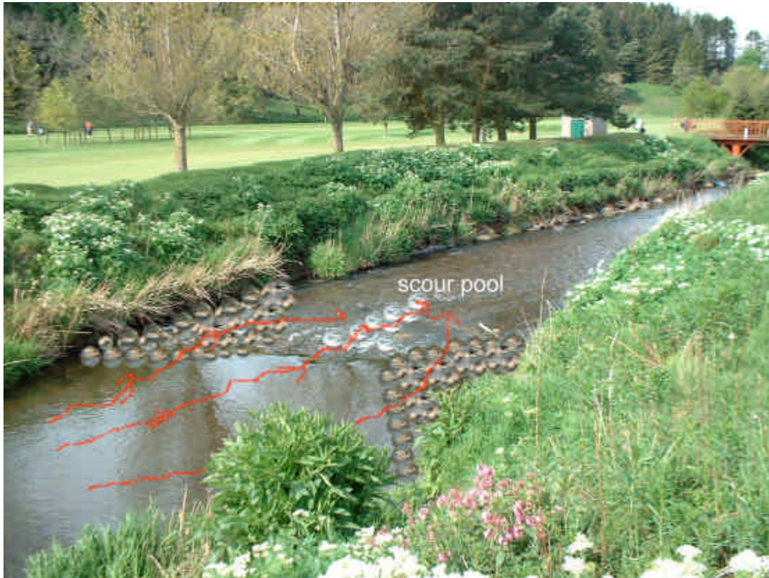
Picture Three – Scour Pool
