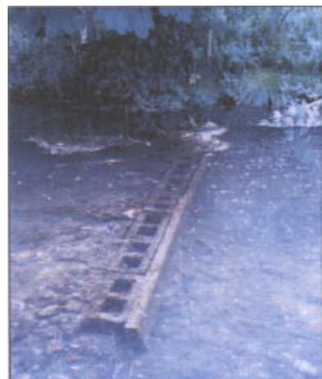
Photo 2. Breezeblock groin u/s weir 1
