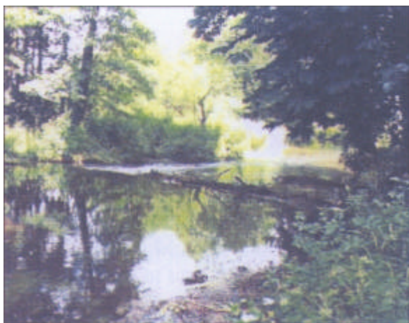
Photo 1. Weir 1 with debris and block groin
