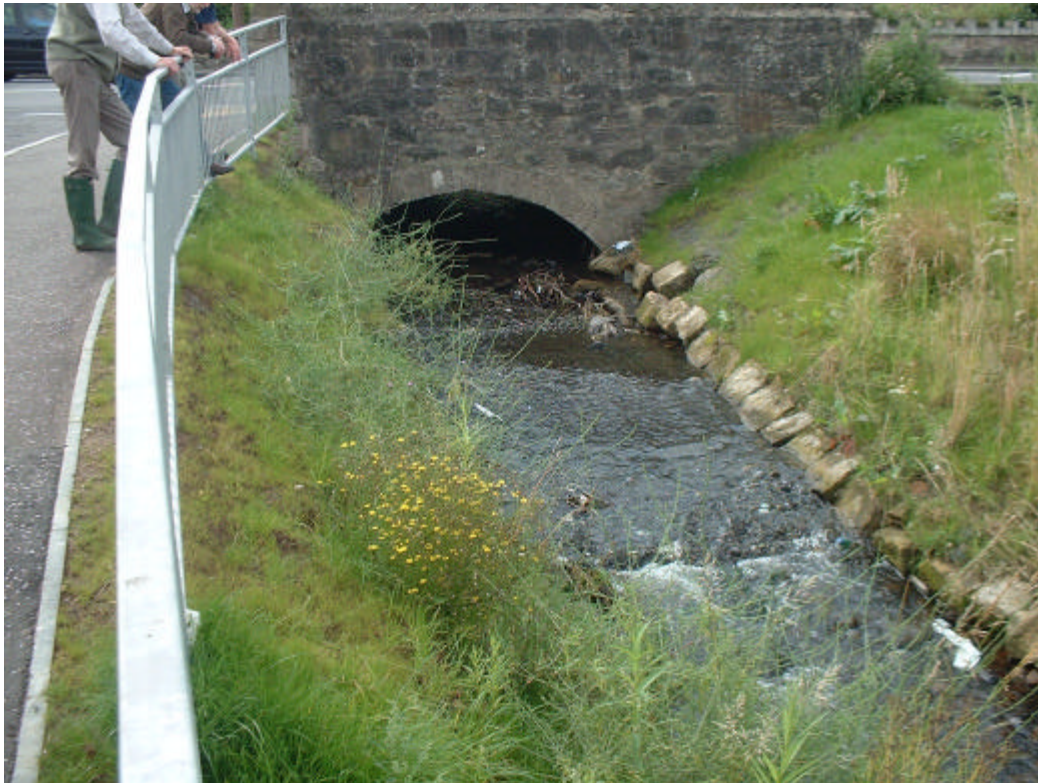
Problem at bridge
