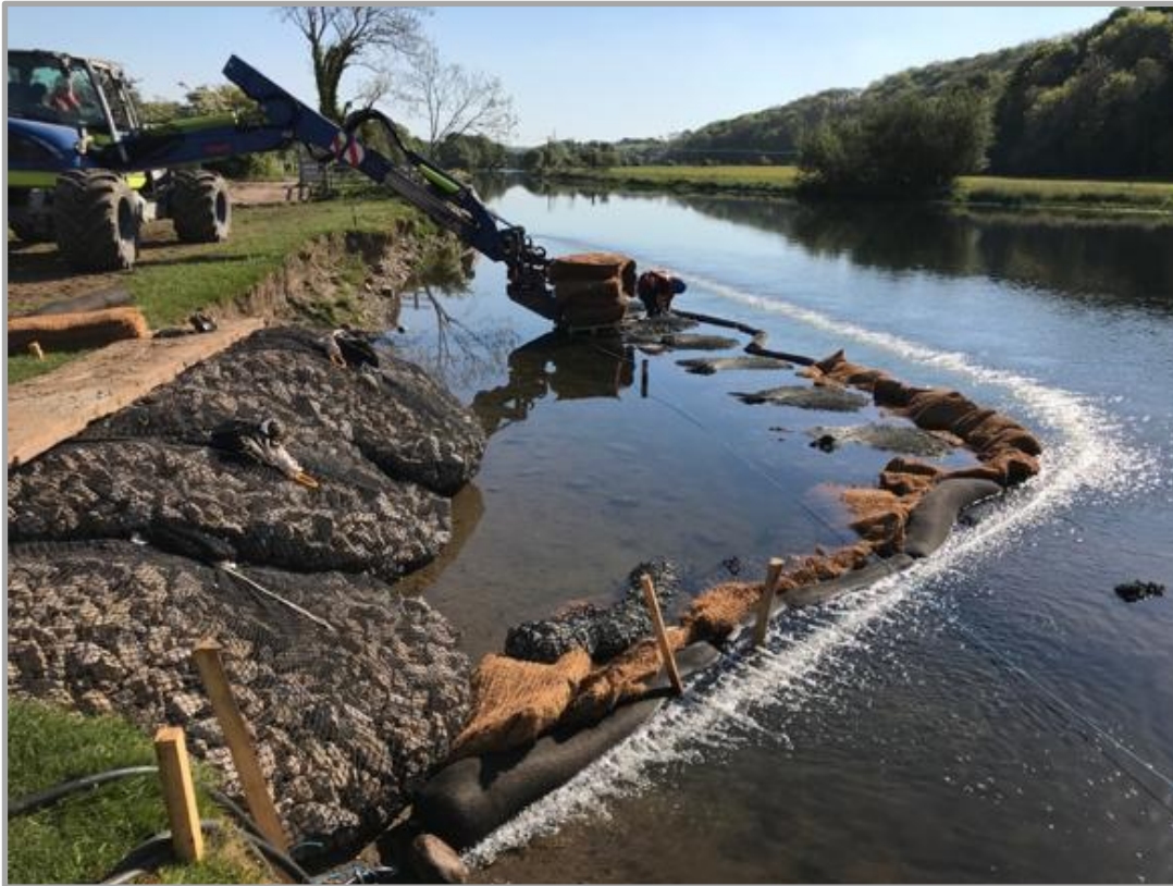
Figure 1 Silt Wattles, Silt Mats and Bubble Barrier to control sediment release (Photo courtesy of Frog Environmental).
