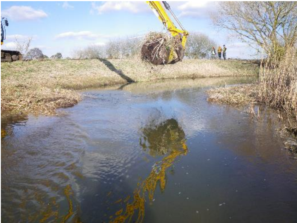
Treatment. Extend the width of the inside of the bend and install a D&D feature.
