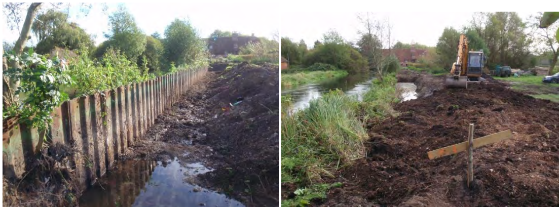
Steel piling exposed prior to removal. Piling removed and bank being profiled
